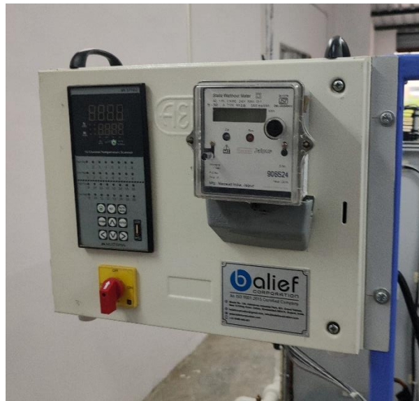
Fig. 6. Control panel for measuring instruments
